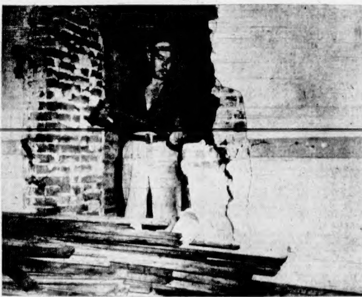
Workmen, armed with crow-bars and wrecking hammers, this week began job of demolishing Government Street buildings to make way for new $2,000,000 Post Office building to be erected on site. Picture shows shows
